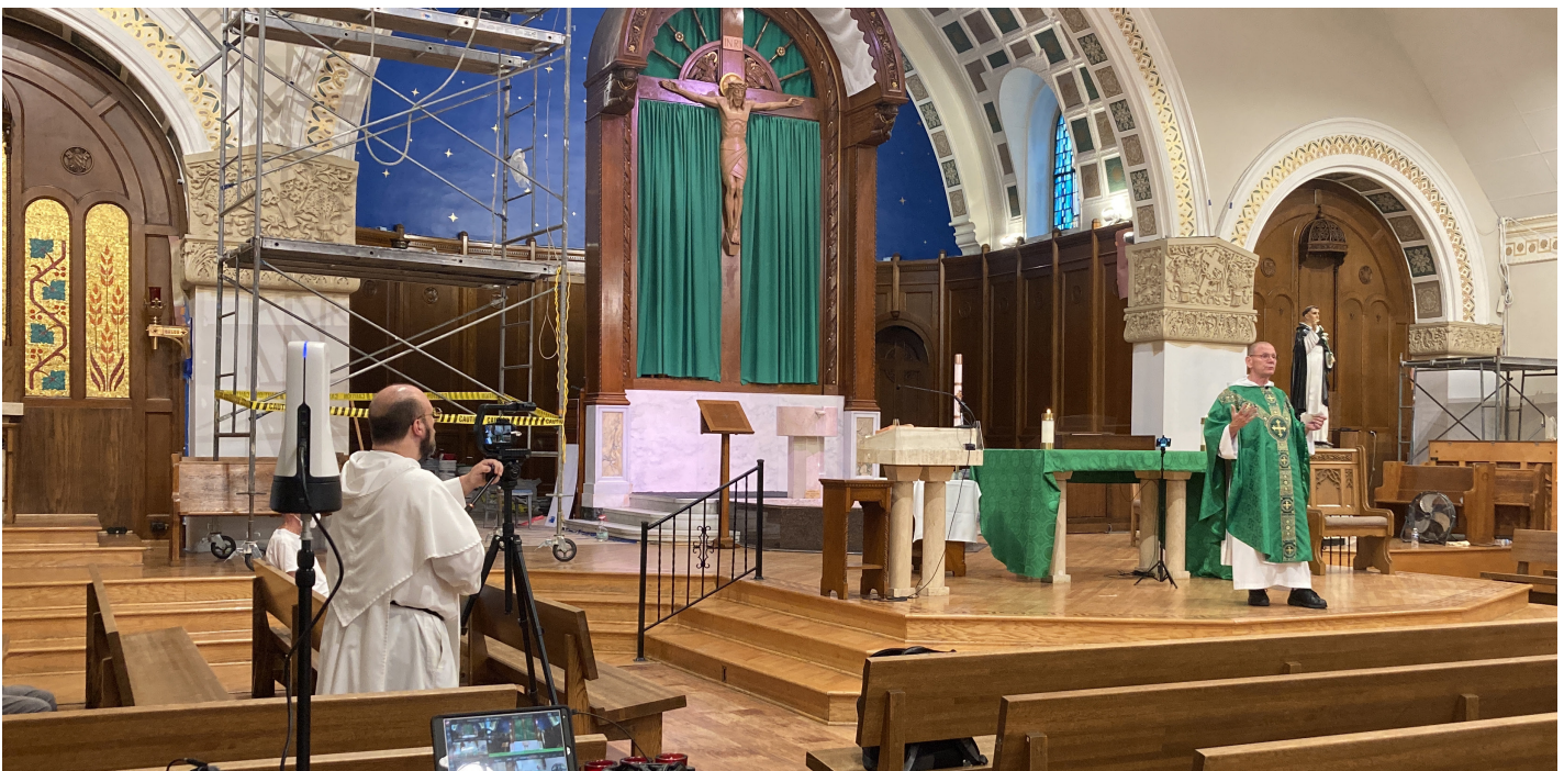
(Page 12) How we make the magic of the livestream happen every Thursday on Facebook and YouTube for our Shrine supporters to join us from around the world. You'll notice the scaffolding, which is part of the renovation taking place at St. Pius V Parish in Chicago, Illinois. (Page 13, Upper left) Close-up of candles with electronic tags; (Upper right) Novena in a box. To light a candle, visit www.candle.the-shrine.org .
